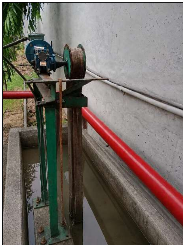
Oil skimmer at Canteen Drain pit
