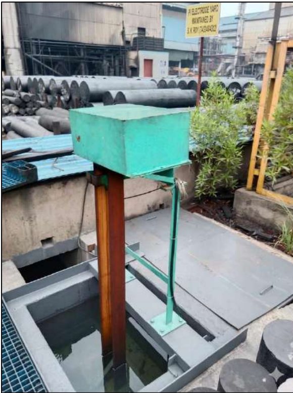
Oil Skimmer PI Area Drain pit
