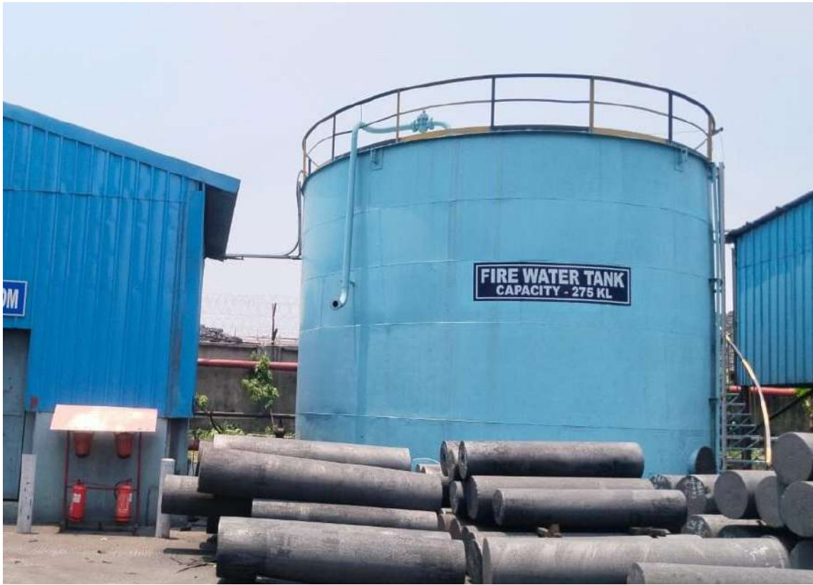
Fire Water Tank
